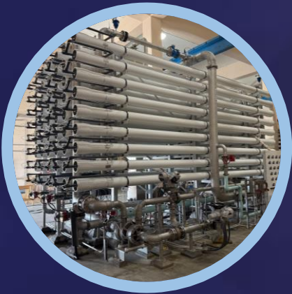
RO Skid 1 Completed 2026
