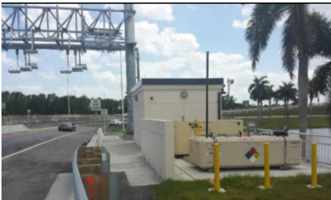
ITS Hub and Tolling Truss
