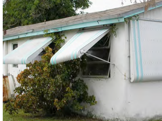
Housing with code problems, Northwest Quadrant
