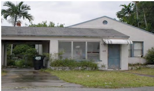
House with code problems, Northeast Quadrant
