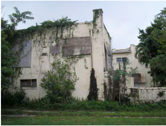
Housing with code problems, Southwest Quadrant
