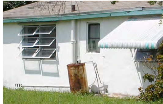
Housing with code problems, Northwest Quadrant
